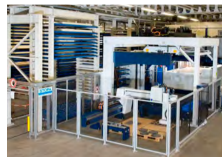
Efficient material flow: Laser cutting system directly connected to the high-bay warehouse.
